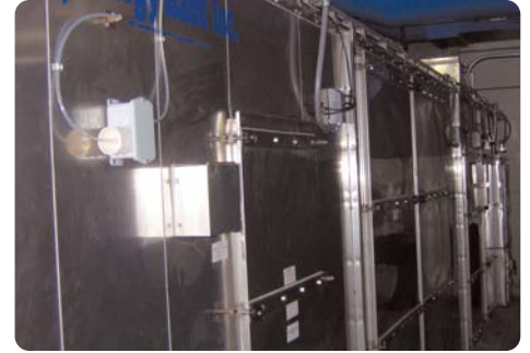
HPscrubber—view of the odor control unit (scrubber) described in the article.
