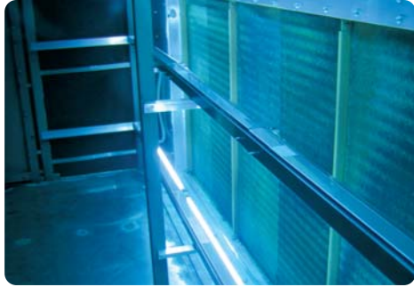
A view of the coils with the UVC lights on.
