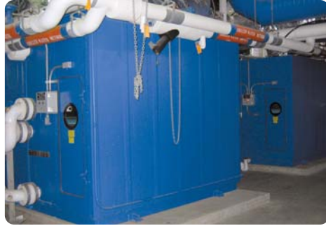
A general view of the mechanical equipment room showing two of the air handlers.
